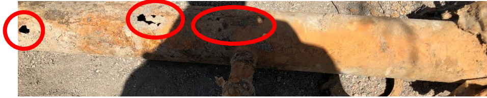
Figure 26: FDC Piping Failure from the Empower Field Fire, Courtesy of FPM Tony Caro
